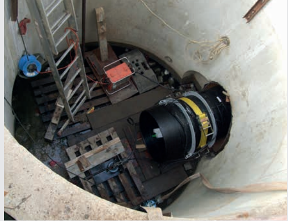
Rehabilitation using short-pipe relining method via shaft installation (PE 100; d 800 mm, SDR 17, module length 700 mm)
