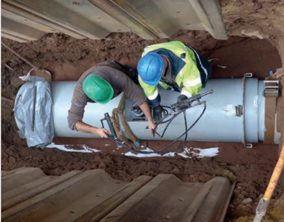
Open-trench pipe laying with sand bed and trench boxes (PE 100 grey/UV-stabilised; d 710, SDR 17.6)
