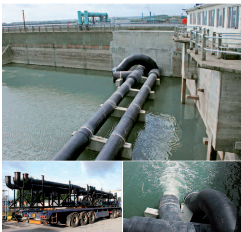
Feed lines made with large-size SIMONA® PE 100 pipes; Welded pipe sections prefabricated at the factory using PE 100; Brackish water storage tank with PE 100 feed pipe, OD 1000/1200 mm
