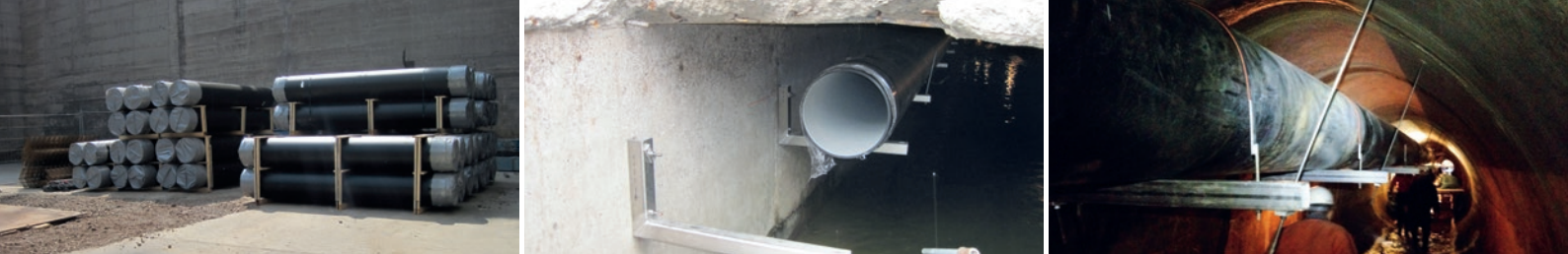
From left to right: SIMOFUSE® pipes in storage; special brackets and supports for the SIMOFUSE® pipes; suspended pipe in ovoid duct
