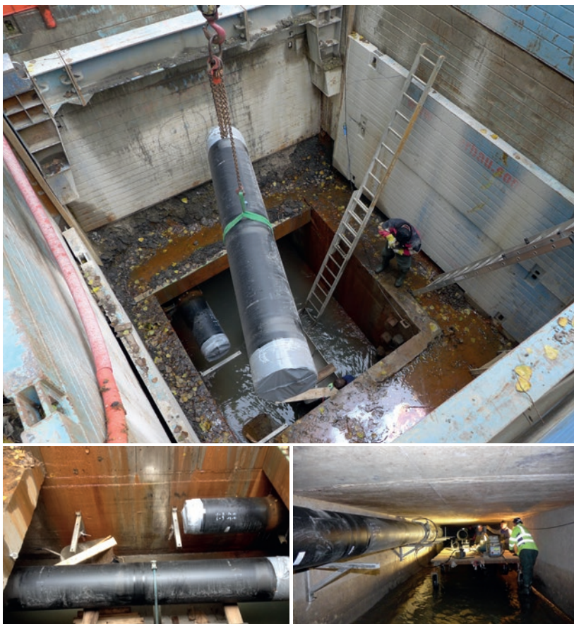
Top: Sinking the SIMOFUSE® pipe modules via the access structure. Bottom left: Transporting the pipe modules on specially built trolleys. Bottom right: Mounting the SIMOFUSE® pressure pipeline in the underground stream section
