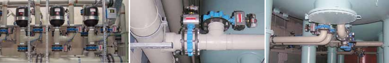
From left to right: Raw water filter system; branch bypass; outlet and regeneration line
