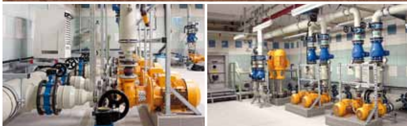
Top: Facility building of Trollmühle Municipal Water Board; Bottom left: Set of pumps for water softening; Bottom right: Regeneration and bypass pumps.
